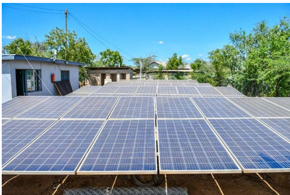
Figure 20: Okapi Green set up this solar array to provide cost effective electricity in Kakuma 3. Photo Credit: JRS
