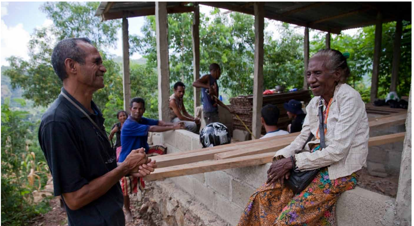
Timor-Leste: Isidoro Costa, JRS Director, visits the house of Rita Indau, for which JRS provided the building supplies while the community offered the labour. 📷 Don Doll SJ/JRS
