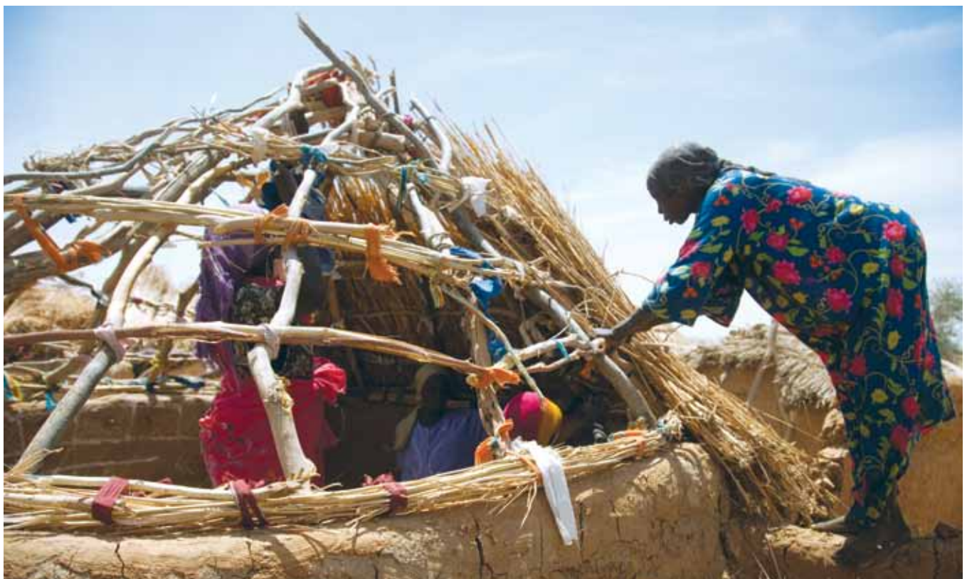
Chad: Constructing the roof of a room in Kounougou refugee camp. (Don Doll SJ/JRS)
